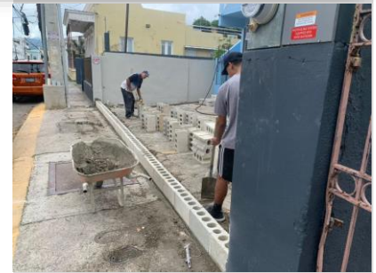
Building a wall in Ponce to create a single entrance to the buildings
