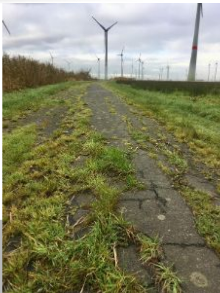
Grass growing through concrete Germany, 2017
