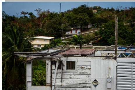
A home damaged by Hurricane Maria in 2017
